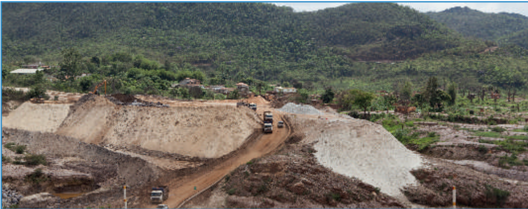
Construction of dam S3 at the settlement of Bento Rodrigues. S3 is a sediment weir, an attempt to reduce the amount of sediment entering the river system from the area of the mine and the collapsed tailings dam. (Nilmar Lage)
